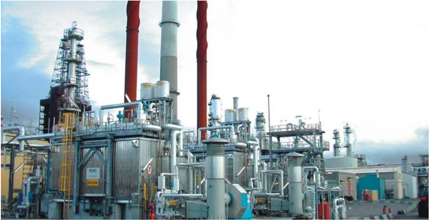
CT "turn-key" thermal power installation 140 t/h for refinery application
