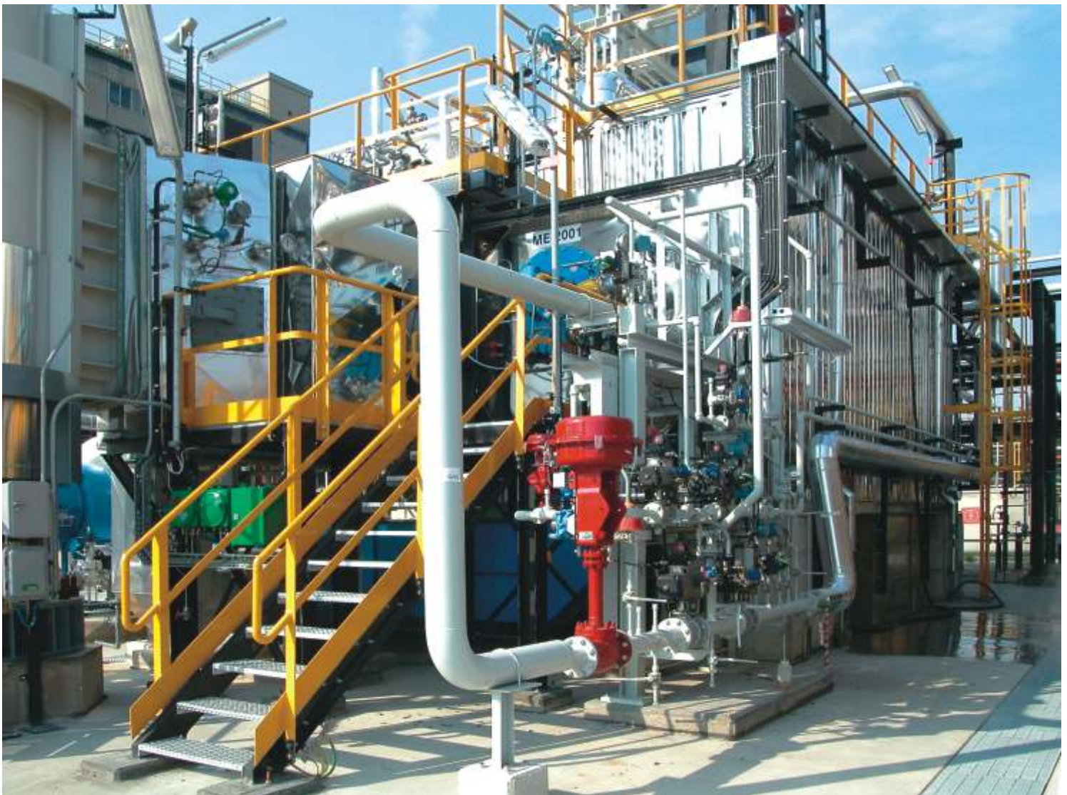
CT Ultra Low Nox application with "reach gas" fuel from chemical process
