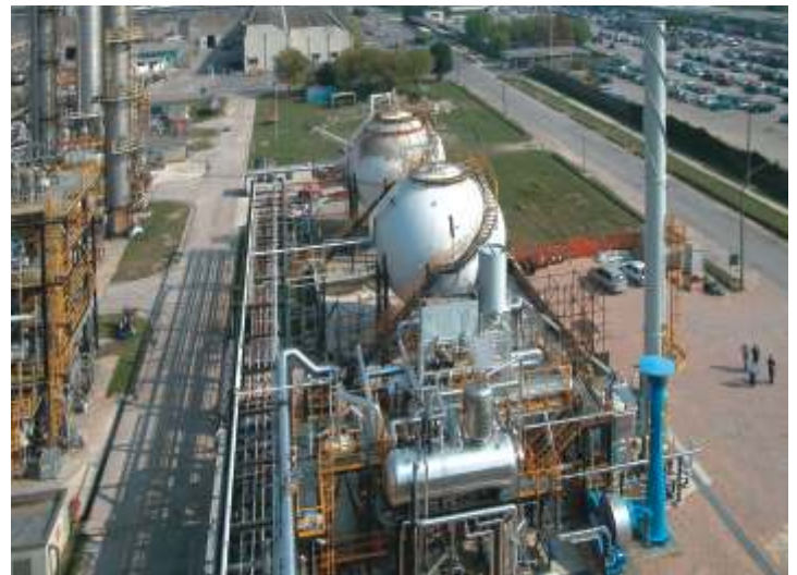
CT "turn-key" installation for chemical application
