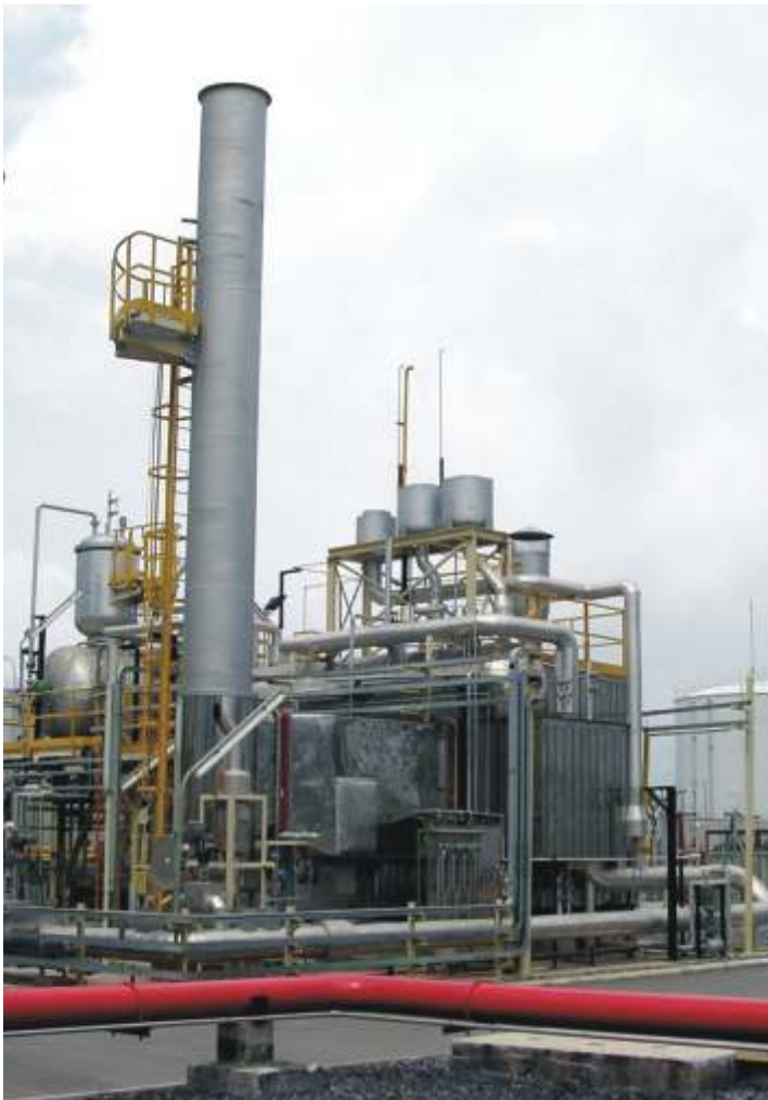
CT 20 t/h auxiliary boiler for power generation
